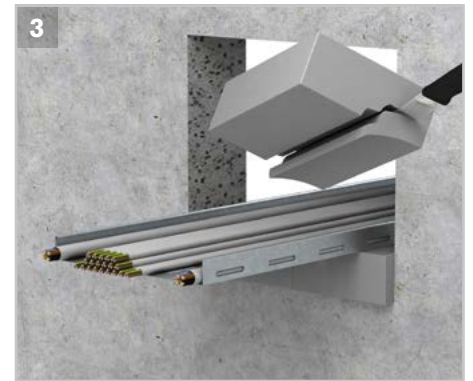
3 Cut out the bricks in such a way, that they lie closely to the cable rack or cables.
